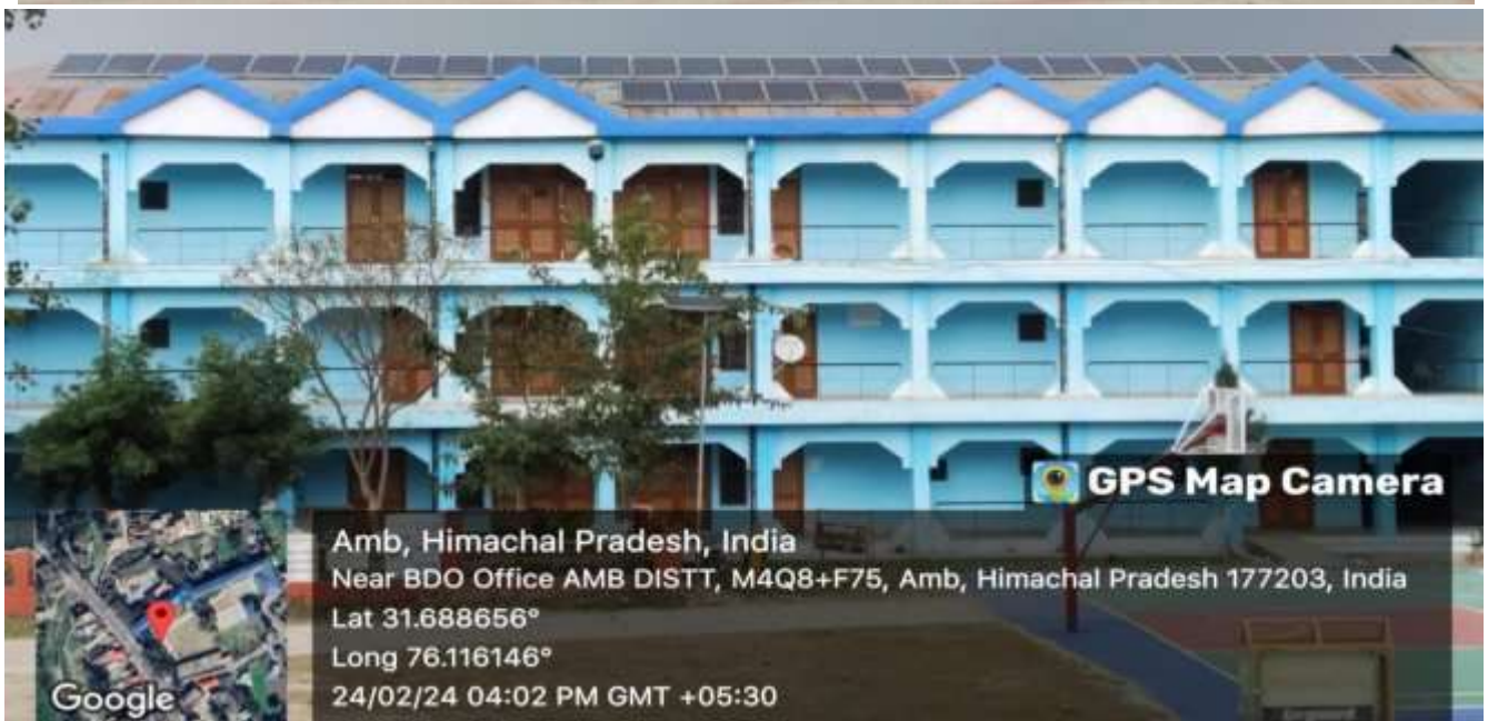
Photos of Solar Panels
